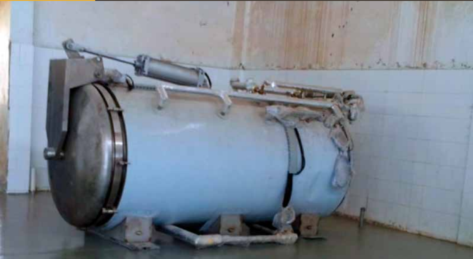
Picture 4 A brand new autoclave in Sana'a HCW treatment centre
