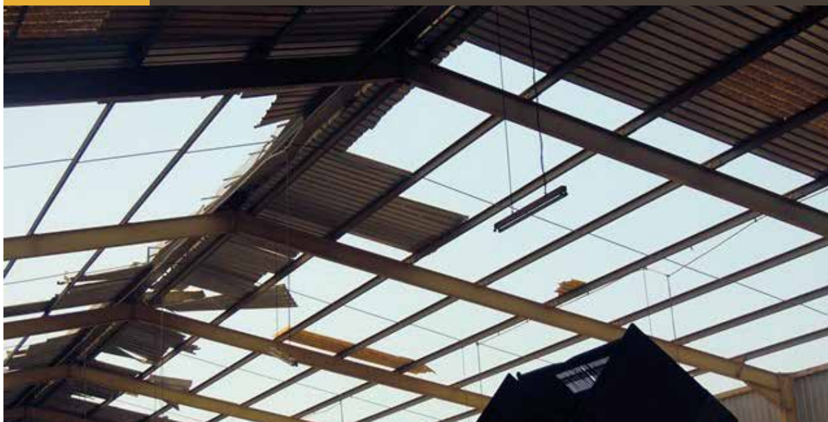
Picture 12 Damaged infrastructure at a recycling plant
